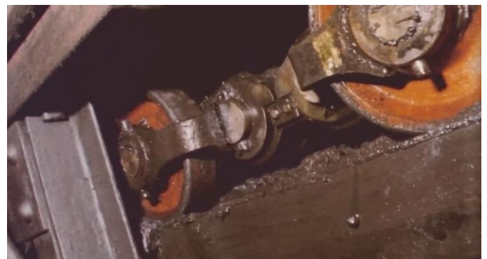
Grease and fibres under the escalators
