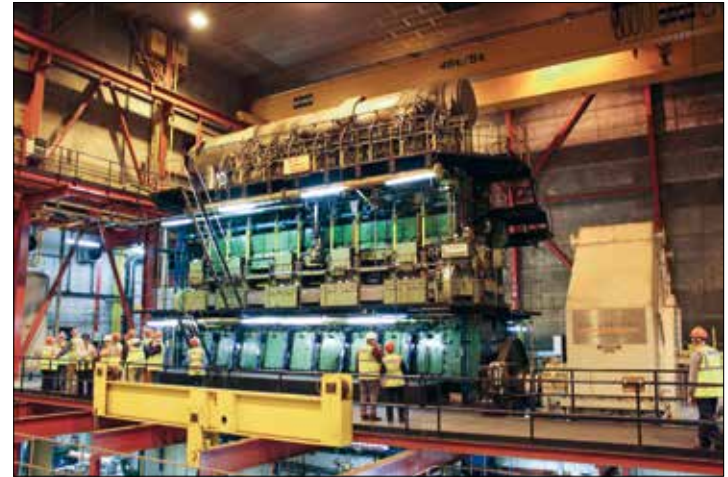
13.19 Guernsey Power Station
