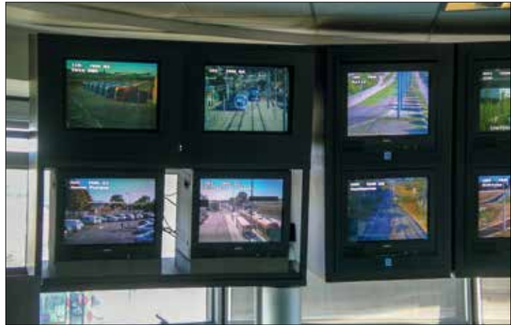
13.03 Tram system control room
