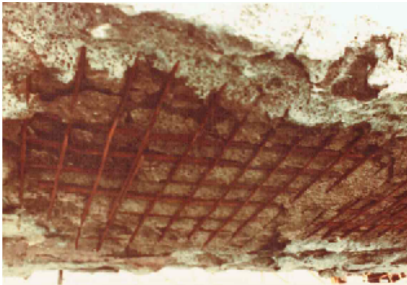
Damaged Concrete showing Reinforcement
