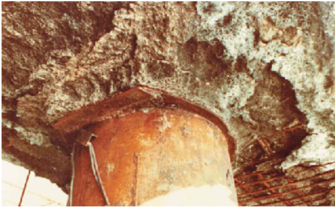
Damaged Underside of Jetty
